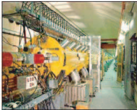
Figure 2.3: The Linear Accelerator Tunnel.
